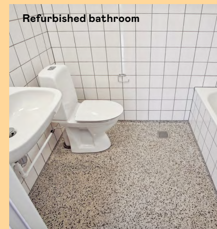
Flawless flooring: hard-wearing, terrazzo has been made with respect to its original design
